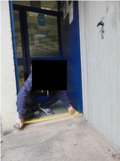
Photo showing the measuring of a door minimum width without the encumbrance of the shutter.
